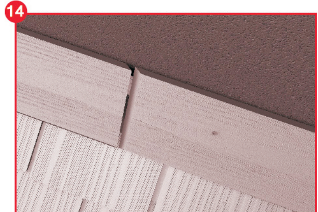
Jointing area shall be chip off 45 degree (as shown in the figure).
